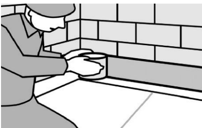
(Fig. 26) The membrane should reach at least 150 mm height on any surrounding walls; the height of the water-bearing level must be observed. Upper edges should be additionally secured with PermaSEAL Overtape. Mineral substrates must be primed with bituminous primer before PermaSEAL Overtape can be applied.
