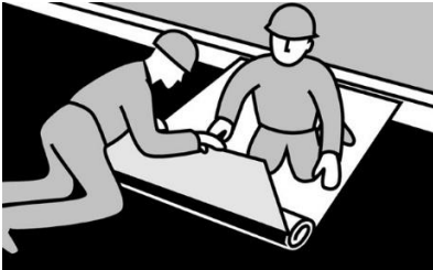
(Fig. 23) Always start laying from the lowest point, working either with or across the gradient. After the sheets have been rolled out and cut to size (we recommend adding an extra of 50 mm), the next step is to align them. Begin by laterally aligning the segments you have trimmed. Next, roll them up again to the middle and cut the backing paper, taking care not to damage the waterproofing layer. Pull off the backing paper slowly and press the sheet down. Next, roll up the other half of the sheet, remove the backing paper, and press the sheet down.
